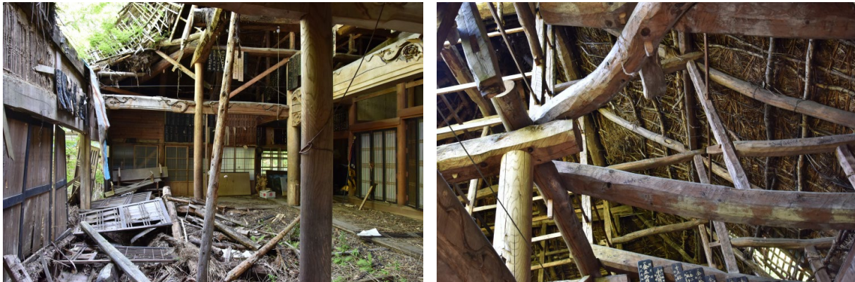
Figures 2, 3 Interiors, debris and roof structure within the temple. Storm damage is exacerbated by snow build-up during the winter months.
