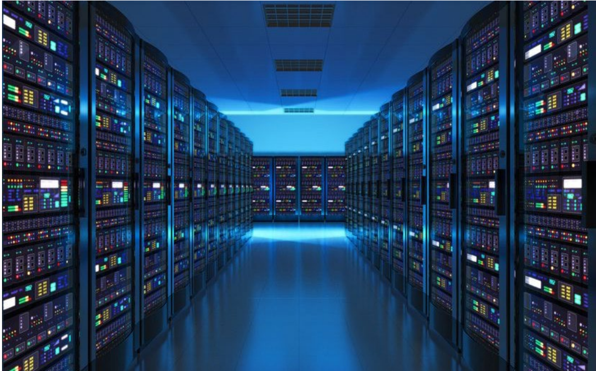
Figure 3 The interior of a Cloud data centre or so-called 'server farm' (Laboratorio Linux, 2017, https://creativecommons.org/licenses/by-nc-sa/2.0/ ).
